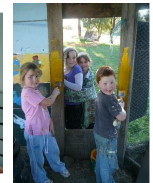
The Little Class are upgrading the chook house, so that it can provide the kitchen with eggs for cooking.
